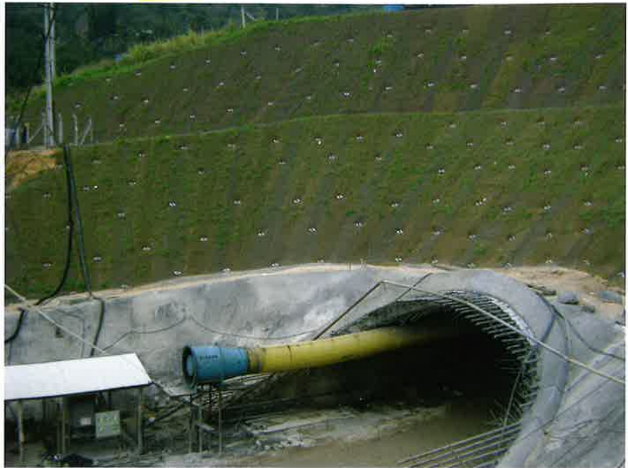
Fig. 1. Tunnel portal with high-strength wire nets in loose ground in Brazil (photo: Geobrugg)
