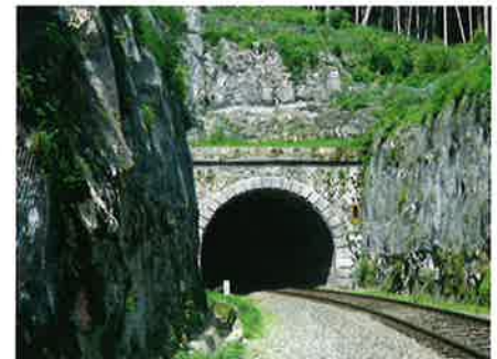
Fig. 3. Securing of a portal and cuttings in rock with nets in Bockenheim, Germany (photo: Geobrugg)
